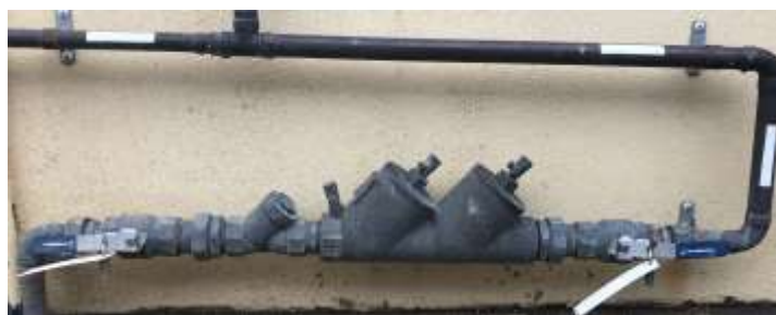
Medium hazard device (Double Check Valve – DCV)
