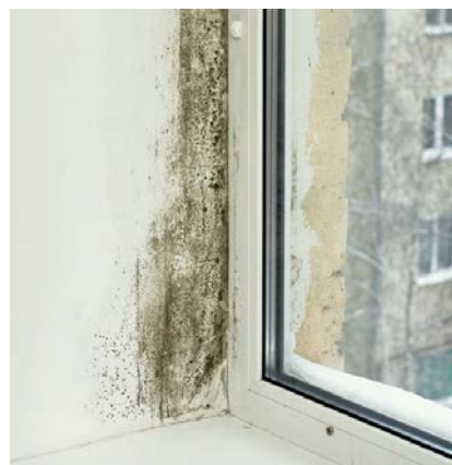
Figure 1 Mould on a wall
