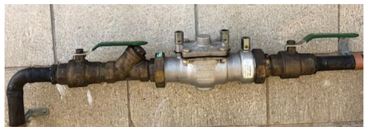
High hazard device (reduced pressure zone device RPZD)
