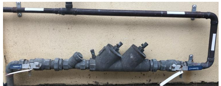
Medium hazard device (Double Check Valve – DCV)
