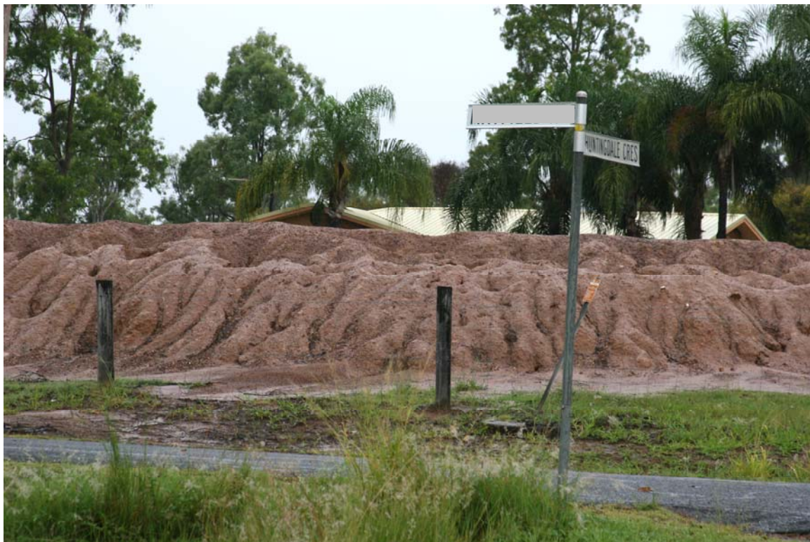
Photo 13. Example of severe erosion of a dam wall in Placid Hills that could be managed by covering the sodic subsoil with topsoil to allow vegetation to establish.
